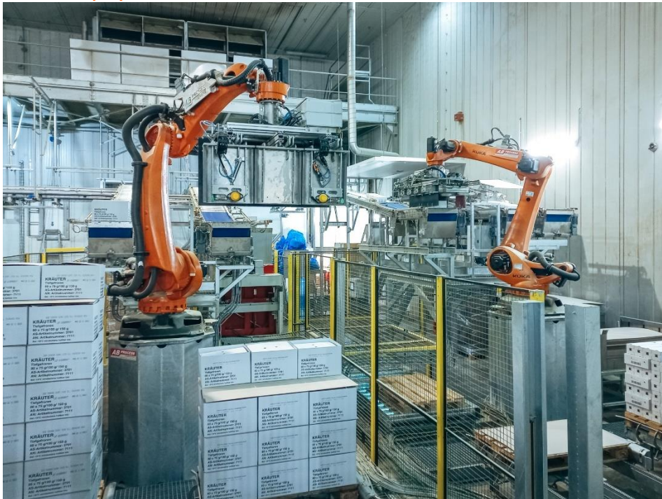
Caption: Impressive palletizing: two KR QUANTEC PA Arctic robots provide automated solutions for low temperatures in the cold-storage room.
